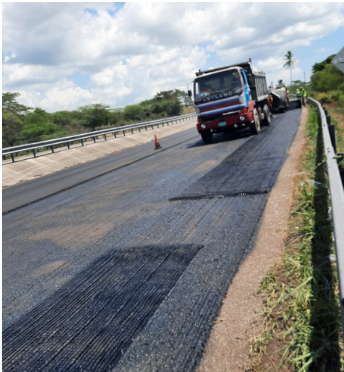
Milled out section at 30+100W being repaved with Geo-grid installed to prevent propagation of cracks
