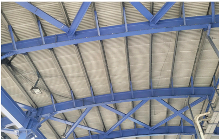
Mesh being installed under canopy to prevent pigeon nesting and defacing toll booths.
