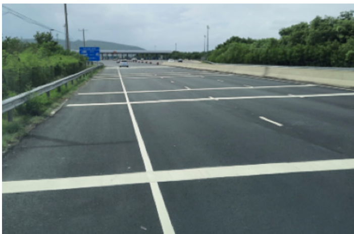
Approach to Portmore Toll after pavement repairs Km4+150W showing lane marking and rumble strips reinstated.
